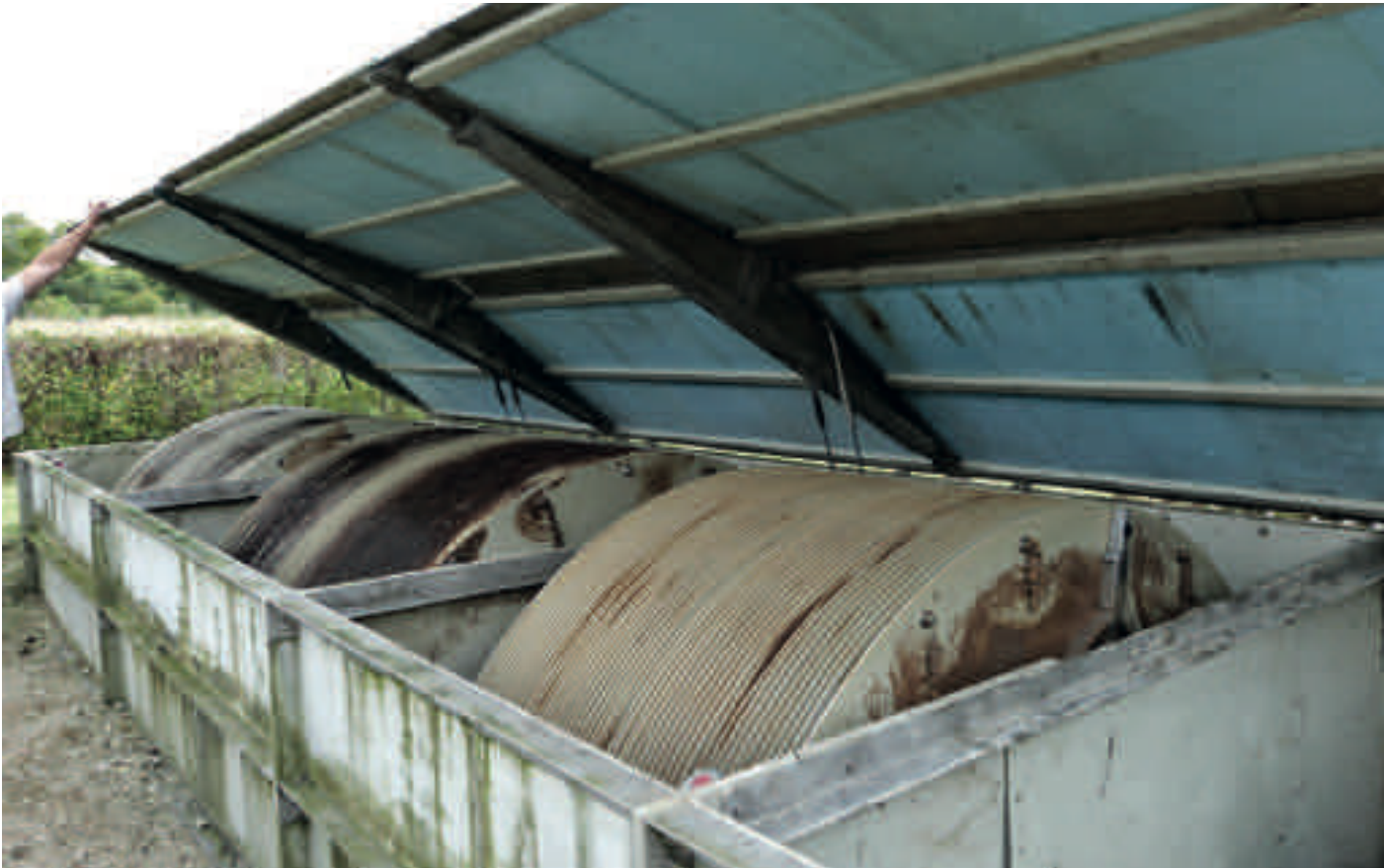
Above: Rotating biological contactors © Roinville-sous-Auneau city
