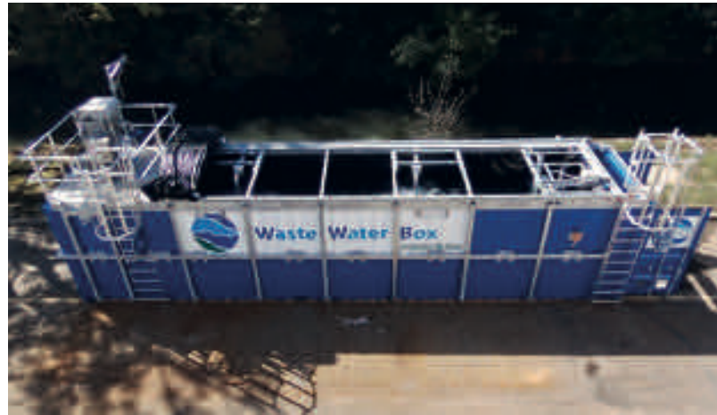
Above: Wastewaterbox containerised plant ©Cohin environnement
