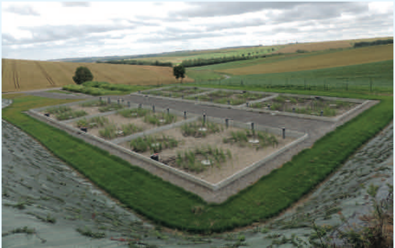
Above: Wastewater treatment plant using reed bed filters at Dohem (62) © AEAP
