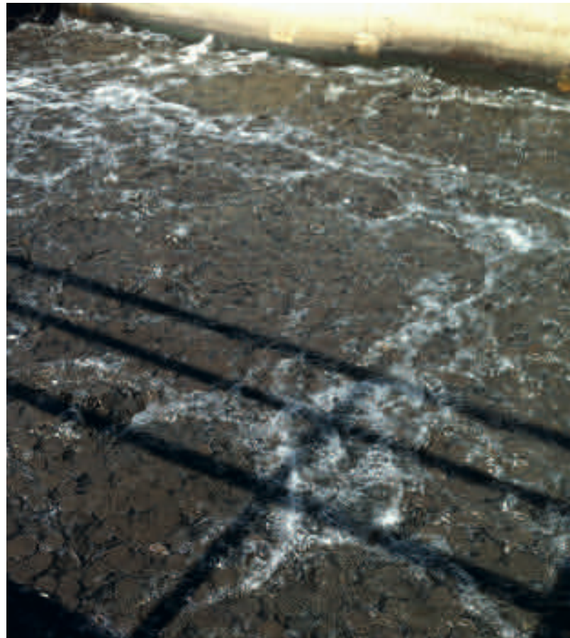
Above: Moving bed bioreactor at the WWTP in Saillon (Switzerland) © Gaël Bost / Surfrider Léman
