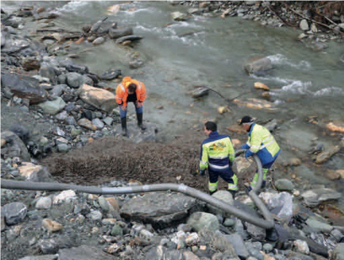
Above: Attempts to recover biomedias lost from the wastewater treatment plant at Evolène © Frank Odenthal
