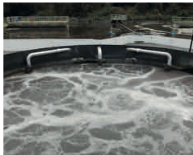
Figure 27 R3F reactor – Quéven WWTP
